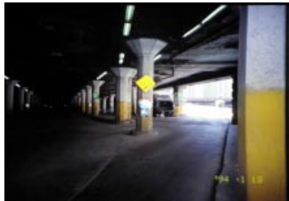
Figure 4: The multi level Chicago 'Walker Drive' and its service roads (Photo taken by the author)
